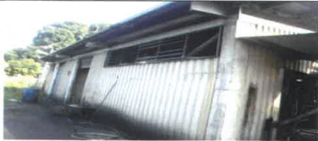
Fig 31.0 View showing broken window frame to be remove and replace with new.
