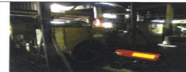
Fig 15.0 View showing Internal view of the Power house.
