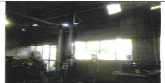
Fig 28.0 View showing internal roofing lining to be remove and replace with new.
