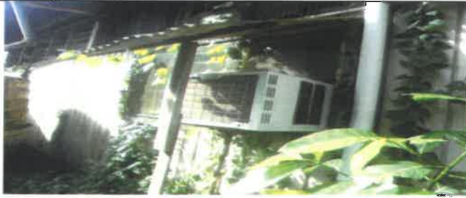
Fig 21.0 View showing faulty air con to be remove and replace with new.
