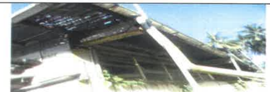
Fig 14. 0 View showing rusty gutters and down pipe to be remove and replace with new.
