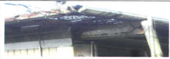
Fig 24. 0 View showing rusty ridge capping to be remove and replace with new .
