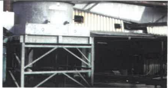
Fig 30.0 View showing frame to be repainted with new silver paint and metal primer.
