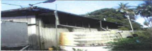
Fig 23.0 View showing all old wall cladding to be remove and replace with new colobond
