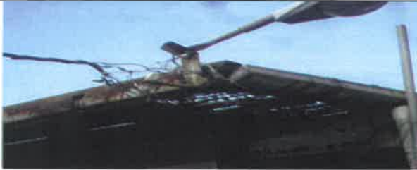
Fig 25.0 View showing security spot light to be remove and replace with new .
