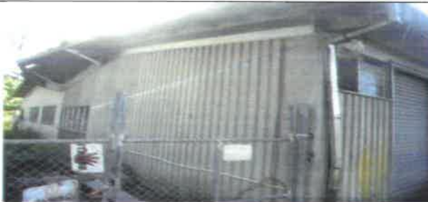
Fig 27.0 View showing old fencing frame to be remove and constructed new fencing.
