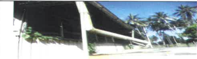
Fig 13.0 View showing old down pipe to be remove and replace with new PVC poly pipe.
