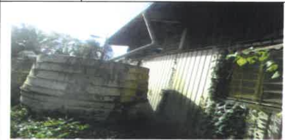
Fig 22.0 View showing old taffa tank to be remove and replace with new.
