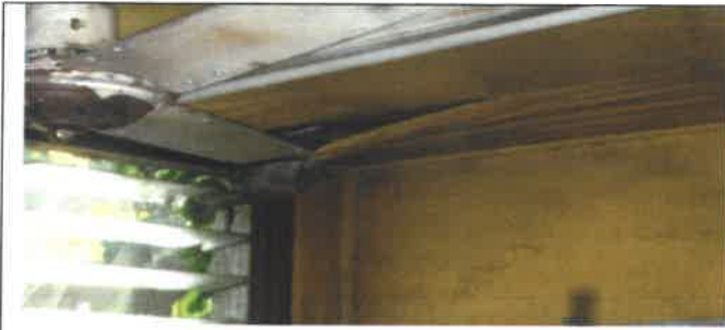
Fig 9.0 View showing rotten ceiling lining to be remove and replace with new.
