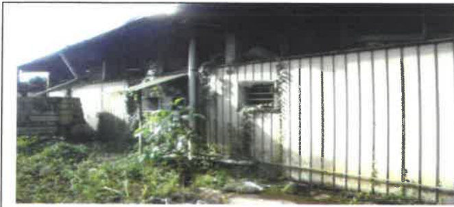
Fig 19.0 View showing shrubs to be cut and remove from the building.
