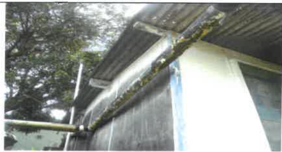
Fig 10.0 View showing wore PVC rain water down pipe to be removed and replace with new.
