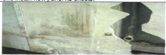
Fig 14. 0 View showing broken fibro to be remove and replace with new.
