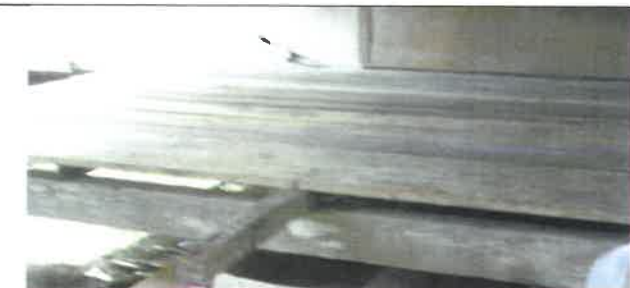
Fig 17.0 View showing rotten floor decking to be remove and replace with new.
