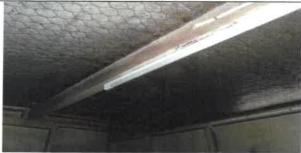
Fig 9.0 View showing faulty ceiling light frame to be remove and replace3 with new.
