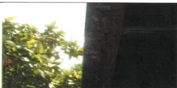
Fig 18.0 View showing rusty gutters to be remove and replace with new.
