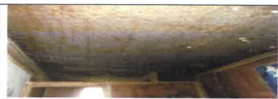
Fig 16. 0 View showing no install of ceiling lining, poor ventilation. Top view of ceiling.
