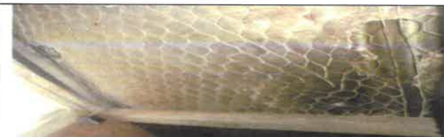
Fig 15.0 View showing wore insect screen to be remove and replace with new.
