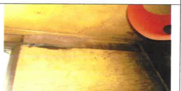
Fig 18.0 View showing rotten wall cladding to be remove and replace with new.
