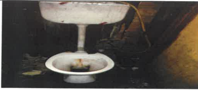
Fig 9.0 View showing faulty Toilet pot, cistern to be remove and replace with new. Toilet room.
