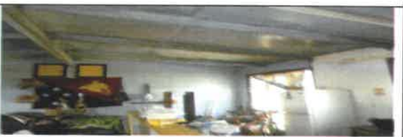
Fig 16. 0 View showing rotten kitchen frame to be remove and replace with new.
