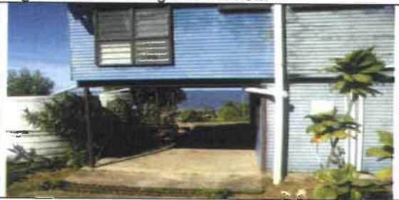
Fig 4.0 View showing old PVC Pipe to be remove and replace with new.
