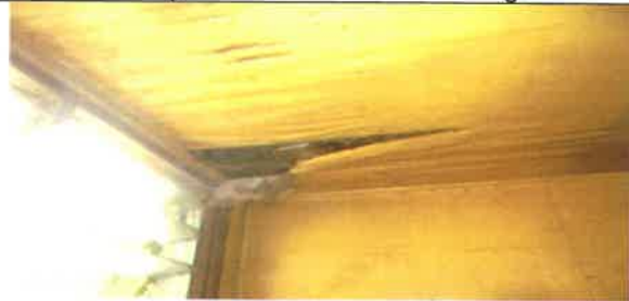
Fig 12.0 View showing rotten ceiling lining to be remove and replace with new. Kitchen
