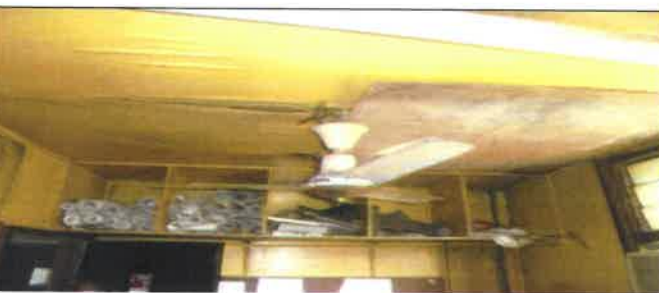
Fig 17.0 View showing faulty fan to be remove and replace with new. Kitchen area.
