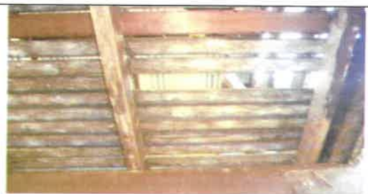
Fig 8.0 View showing rotten flooring to be remove and replace with new.
