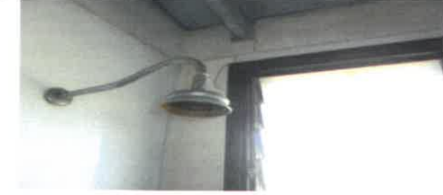
Fig 11.0 View showing rusty rose to be removed and replace with new. Bathroom.
