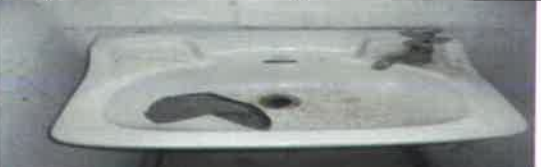
Fig 26. 0 View showing broken hand basin to be remove and replace with new.
