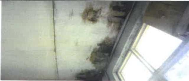
Fig 11.0 View showing rotten ceiling lining to be remove and replace with new.
