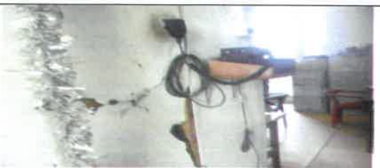
Fig 10.0 View showing rotten wall lining to be remove and replace with new.
