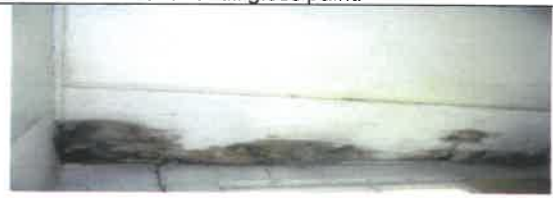
Fig 14. 0 View showing rotten wall lining to be removed and replace with new.
