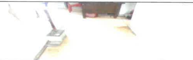
Fig 15.0 View showing wore vinyl tile to be remove and replace with new.
