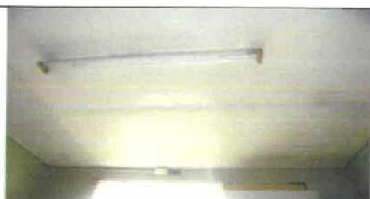
Fig 18.0 View showing faulty light fitting to be remove and replace with new.
