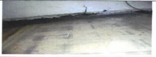
Fig 24. 0 View showing Internal wall lining to be remove and replace with new. Internal partition.
