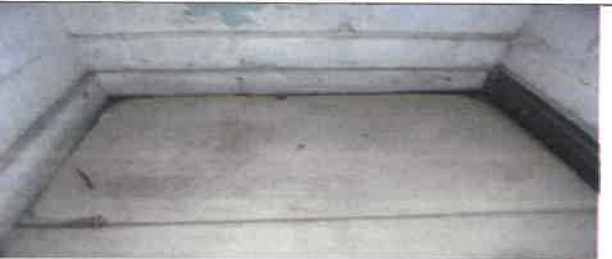
Fig 27.0 View showing no toilet install. Woman's toilet room
