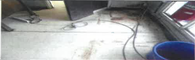
Fig 13.0 View showing wore vinyl tile to be remove and replace with new. All vinyl tiles to be remove and replace with new.
