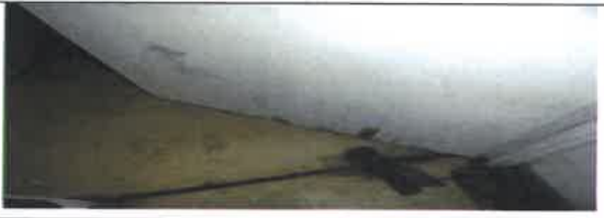
Fig 34. 0 View showing Internal wall lining to be remove and replace with new.
