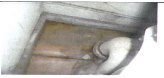
Fig 28.0 View showing poor toilet pot, cistern to be remove and replace with new.
