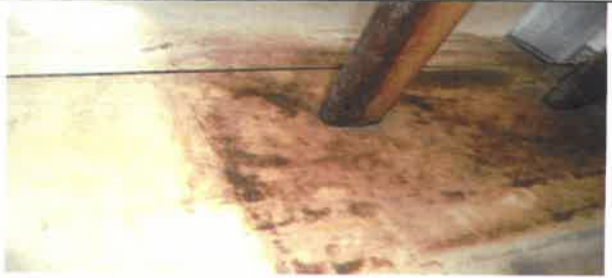
Fig 21.0 View showing wore vinyl tiles to be removed and replace with new.
