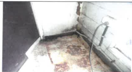
Fig 10.0 View showing wore vinyl roll tile to be remove and replace with new.
