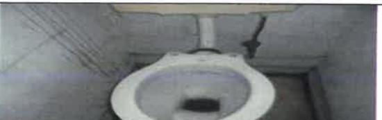
Fig 36. 0 View showing faulty toilet pot to be remove and replace with new.
