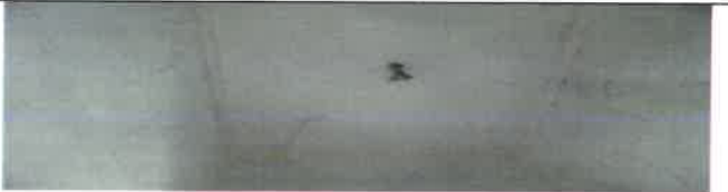
Fig 35.0 View showing faulty light fitting to be remove and replace with new. Corridor light.
