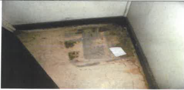
Fig 19.0 View showing wore vinyl tile to be remove and replace with new.
