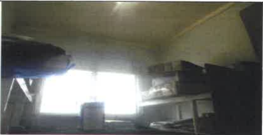
Fig 22.0 View showing poor ventilation, few window fabrication. File section 1 office.
